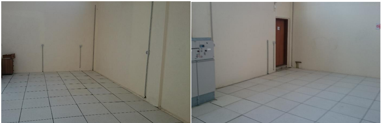
Figure 2-3: Proposed areas for the installation of the voltage stabilizer at NG WWTP
